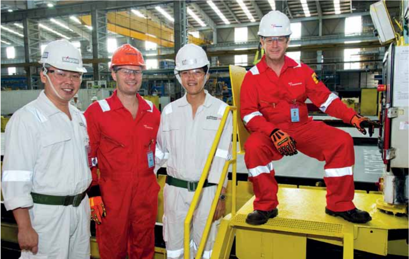
Cutting steel to mark the start of the construction of project B364, a Keppel FELS Super B Class Big Foot jackup rig being built for Transocean Offshore Deepwater Holdings, are (L-R) Mr Chris Ong Leng Yeow, Acting Executive Director of Operations, Keppel FELS, Mr Douglas Brown, Project Manager, Transocean, Mr Shawn Yeo, Project Manager, Keppel FELS and Mr Sylvian Lalycan, Senior Electrical Engineer, Transocean
